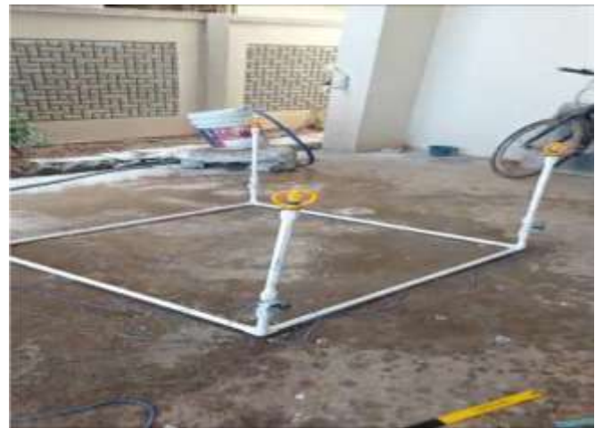
Fig. 9. Field pipe network with PVC pipes, solenoid valves and sprinkler risers.
