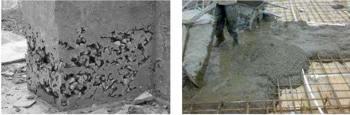
Figure No. 3.3 Segregation of Concrete
