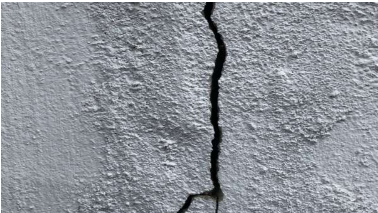
(Figure 1 & 2: Examples of typical concrete cracks in civil structures, highlighting the need for automated detection.)
