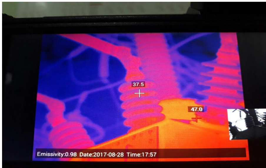
Figure 6: hot spot cleared on Y phase Bushing
