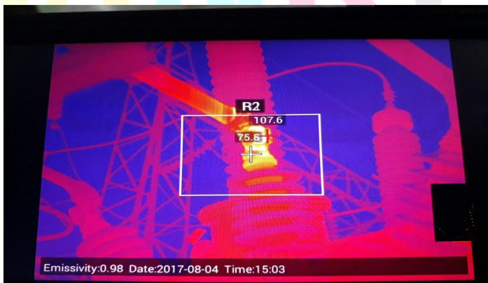
Figure 2: Hot spot on 132kV Y phase bushing
